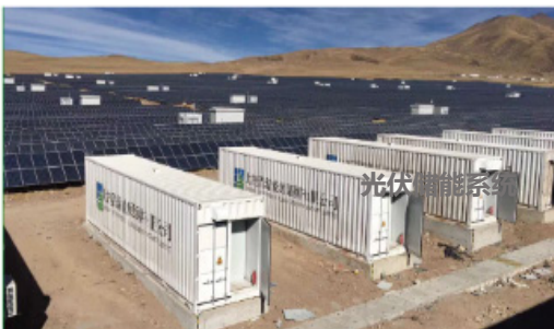
Photovoltaic and Battery Energy Storage System
