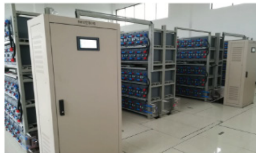
Active Distribution Network Battery Energy Storage System
